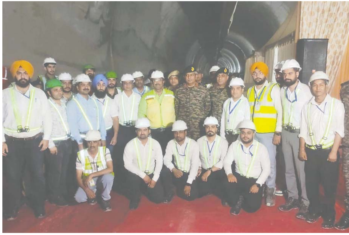
JAMMU, BRO officers along with other officials at the Sungal Tunnel on Akhnoor-Poonch National Highway in Jammu on Tuesday. UNI
